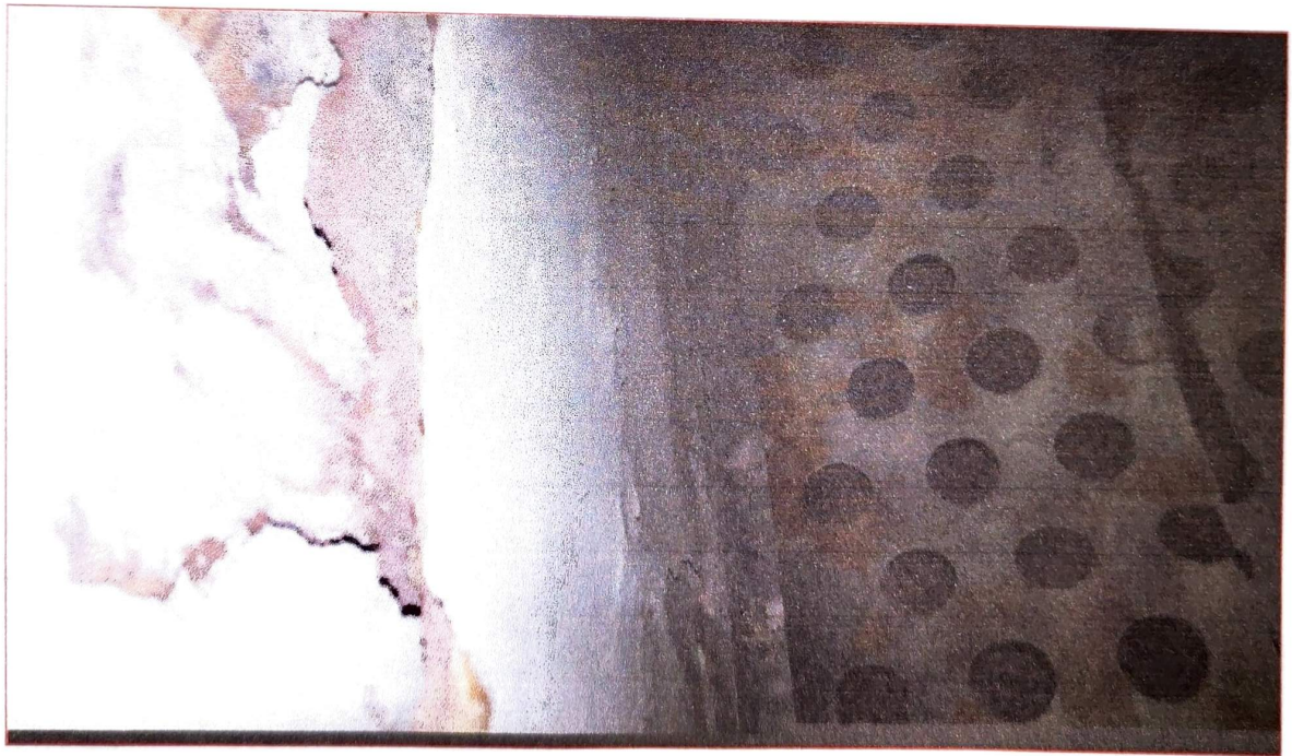
Corrosion of GD screen & ESP casing due to acid condensation.
