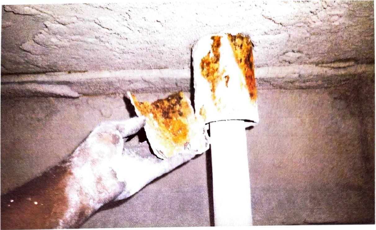
Typical corrosion in ESP supports.
